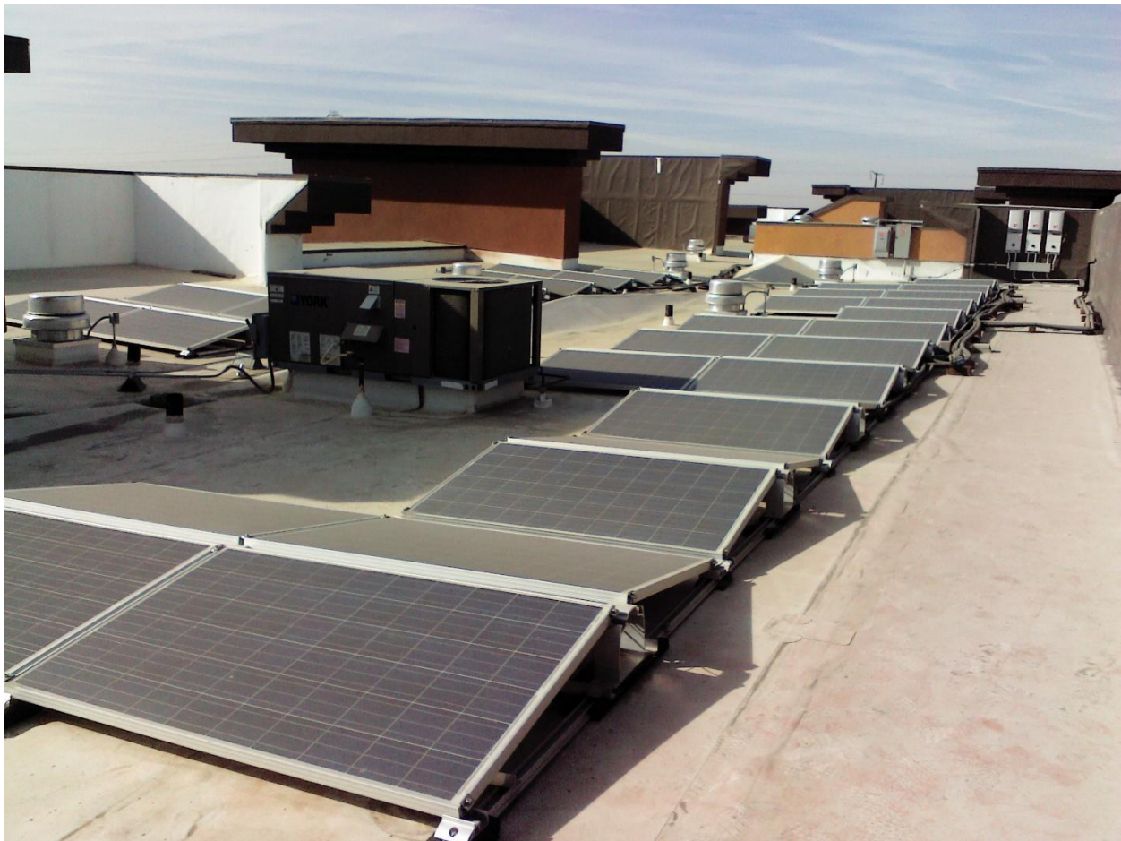
SunDrum® Solar HarvestHP™ Hybrid PV/T-HP Array on Hotel Roof
